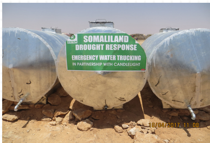
Water tanks installed in Sabawanaag village
